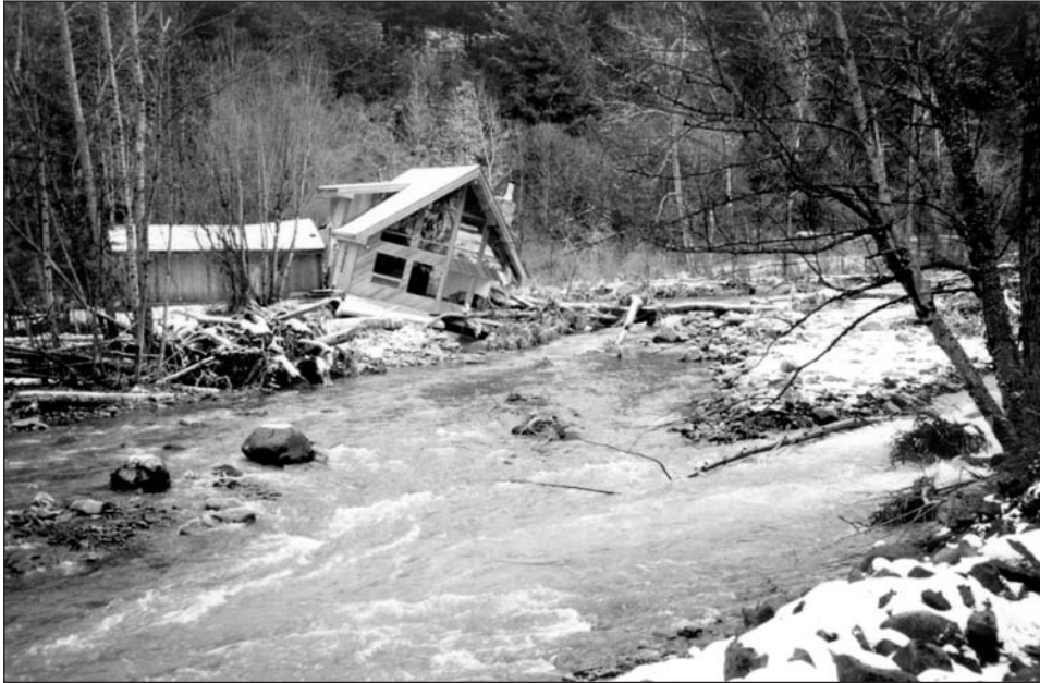
Figure C-7. Home damaged along a stream subject to flash flooding due to surrounding mountainous terrain.
